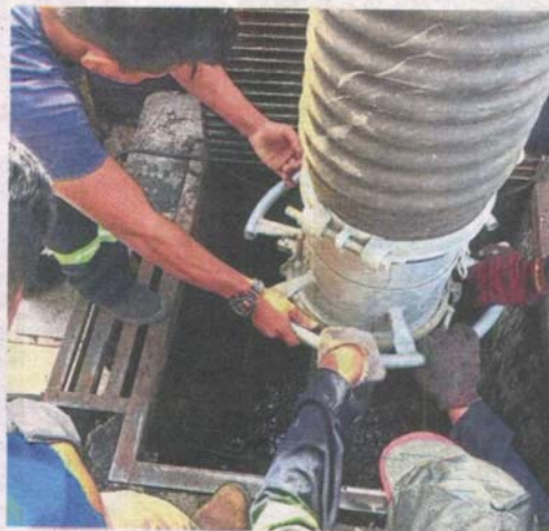
Workers using a vacuum suction pipe to remove silt in the sump at Dataran Templer.
